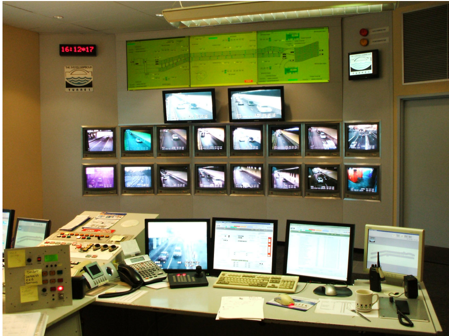
Photograph 1 SHT control room.
